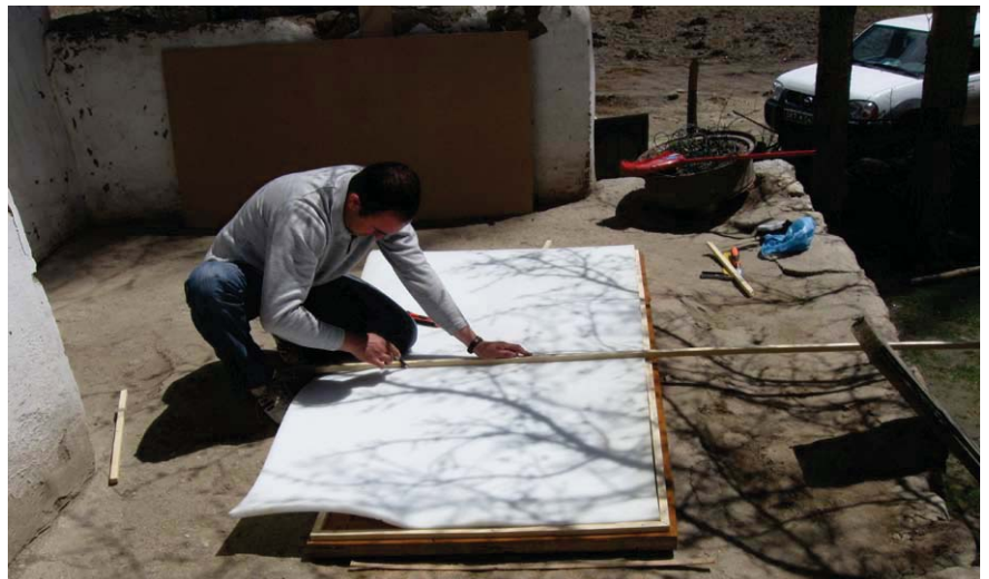
An old door is covered with insulation material in a village in Gorno-Badakhshan. In some cases, this is a viable alternative to the installation of a new door.
