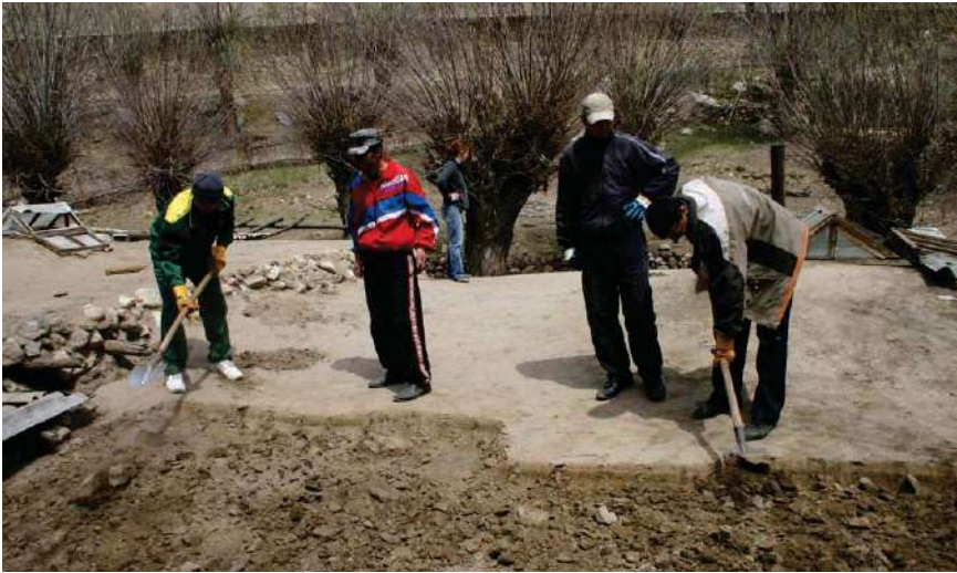
Construction workers are working on the insulation of a roof in a village in Gorno-Badakhshan.
