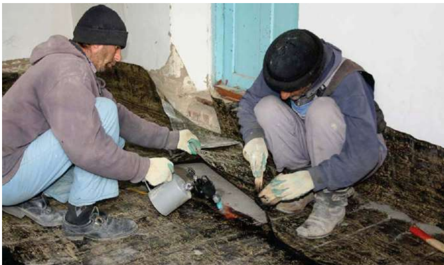
A team of two construction workers is working on the insulation of the floor in a house in the town of Murgab, Gorno-Badakhshan.
