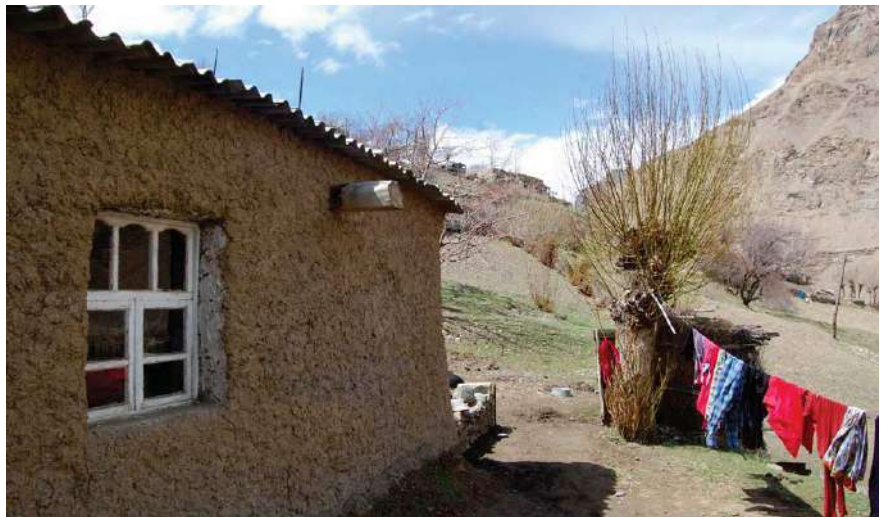
A typical Pamiri house in the village of Barvoz in Gorno-Badakhshan. In spite of the long periods of cold in winter, single-glazed windows are still quite common in the region.
